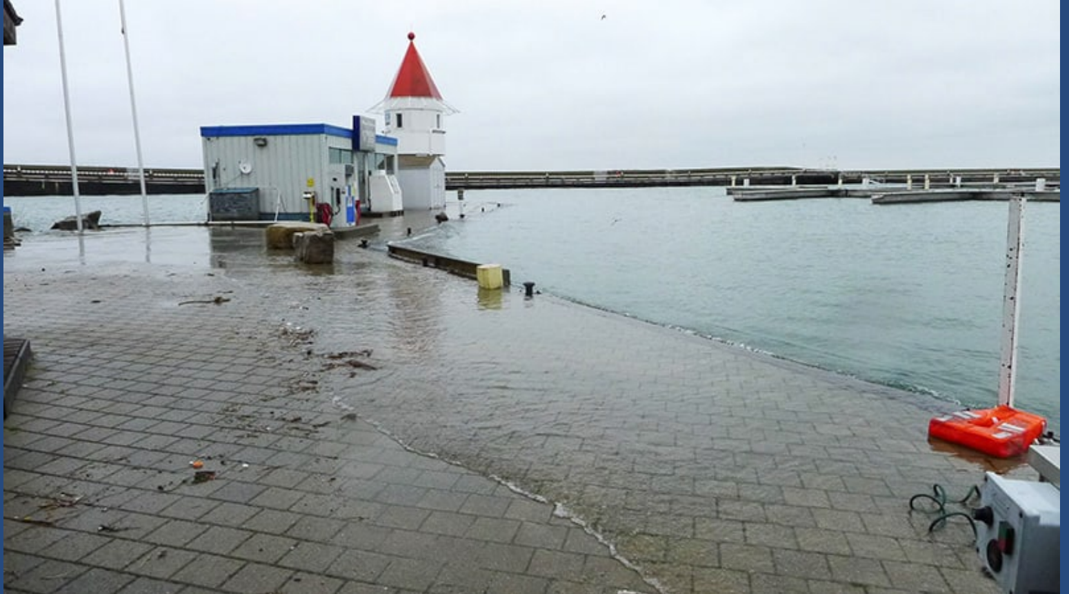
Recent flooding on site
