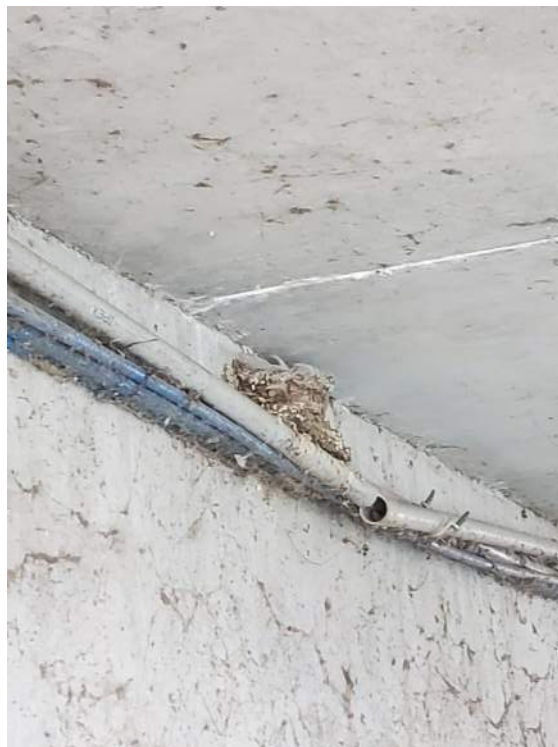
Figure 112: View of a Barn Swallow nest on cables in the unnamed concrete bridge northwest of Bridge 2 (B2). June 23, 2022.
