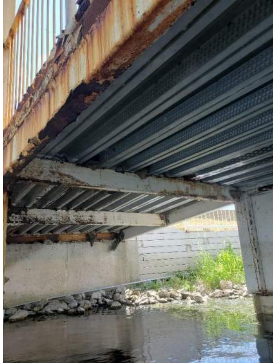
Figure 53: View, facing southeast, of prevalent Barn Swallow nesting under Secondary Tower Ramp Element 7 (SB7) at Cinesphere (B92569). June 23, 2022.
