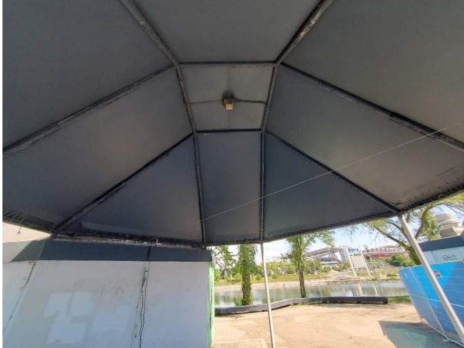
Figure 21: View, facing north, of the canopy between the Commons North Washroom (B92543) and the Dry Storage Building (B92542). June 20, 2022.
