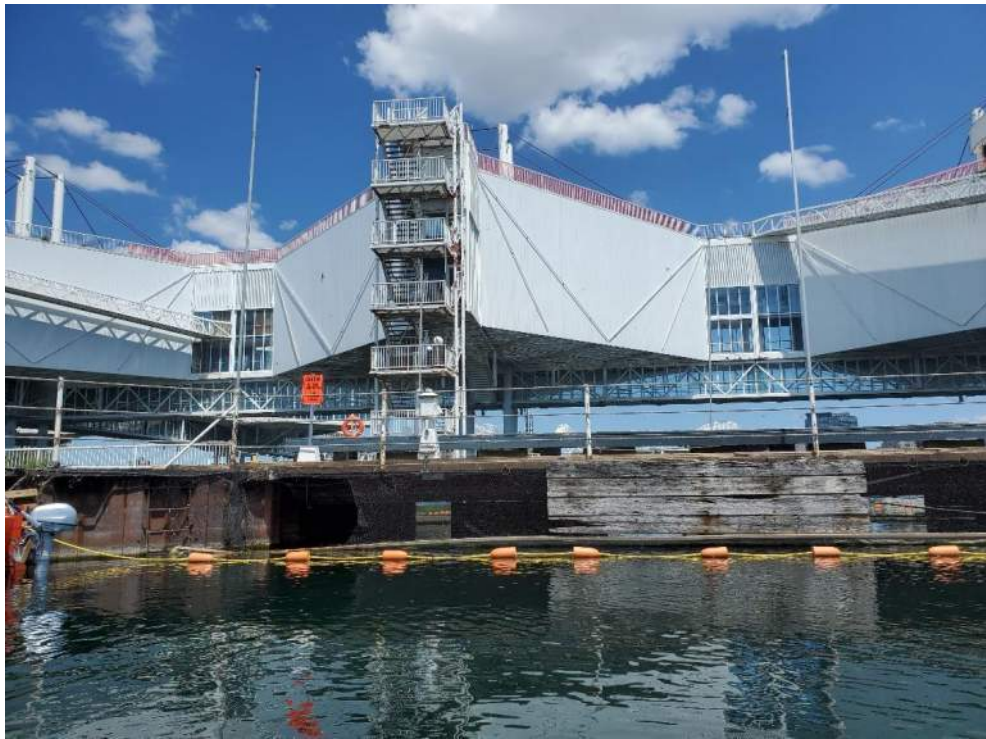
Figure 74: View, facing north, of Bridge 5 (B92575) and Pods 3-5 (B92549-3, B92549-4, B92549-5), providing nesting areas for Barn Swallows and Cliff Swallows, respectively. June 23, 2022.
