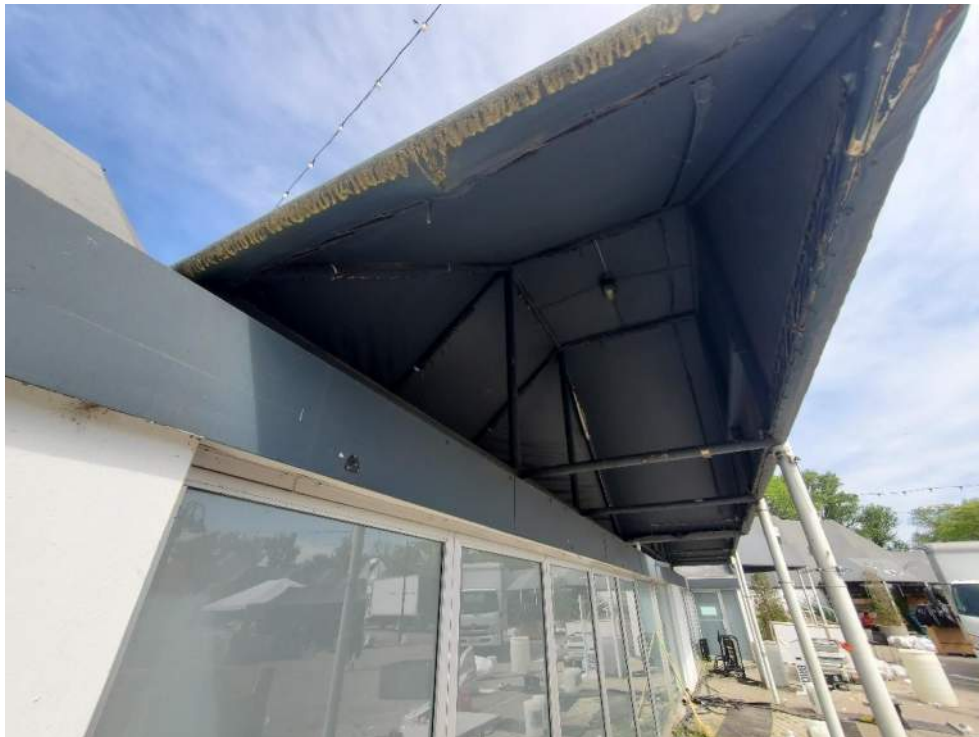
Figure 16: View of canopy on Commons West Building (B92546) where Barn Swallows nest. June 20, 2022.
