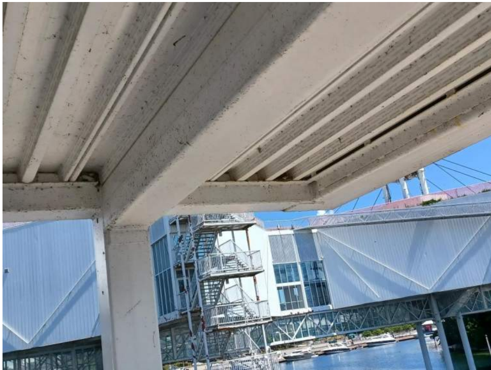
Figure 54: View of Cliff Swallow nests in grooves in underside of Secondary Tower Ramp Element 7 (SB7). June 23, 2022.
