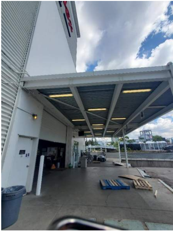
Figure 118: View, facing north, of the loading docks on Live Nation grounds. July 12, 2022.
