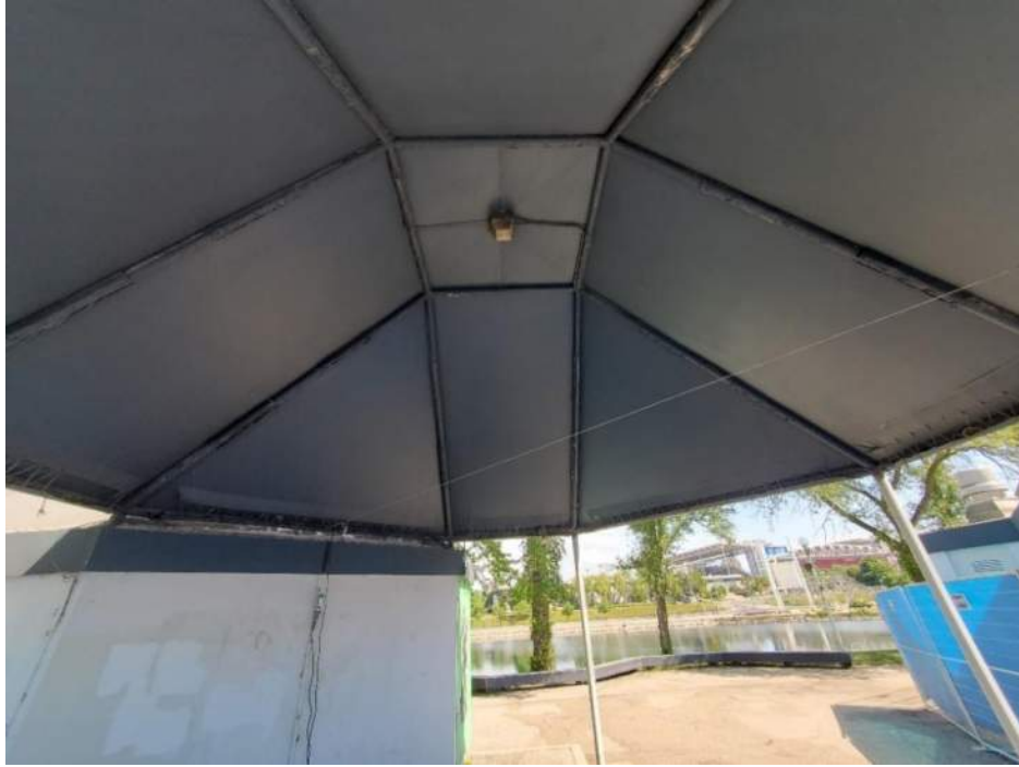
Figure 21: View, facing north, of the canopy between the Commons North Washroom (B92543) and the Dry Storage Building (B92542). June 20, 2022.
