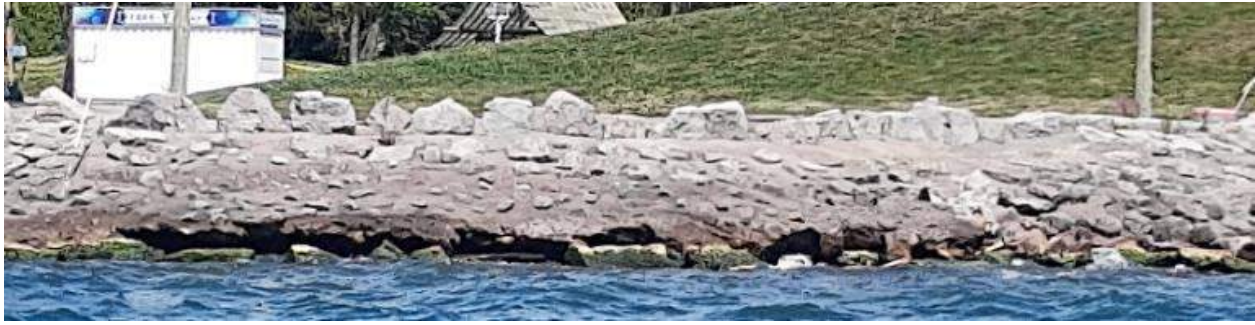
Figure 12: Deterioration of grouted stone revetment at east headland (from Jacobs, 2020)
