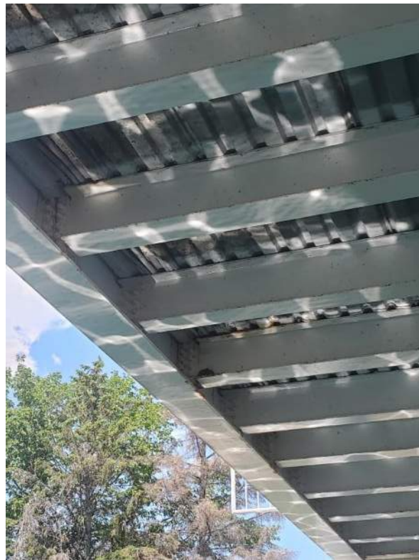
Figure 126: View of a Barn Swallow nest on a girder on Bridge 1A (B1A). June 23, 2022.
