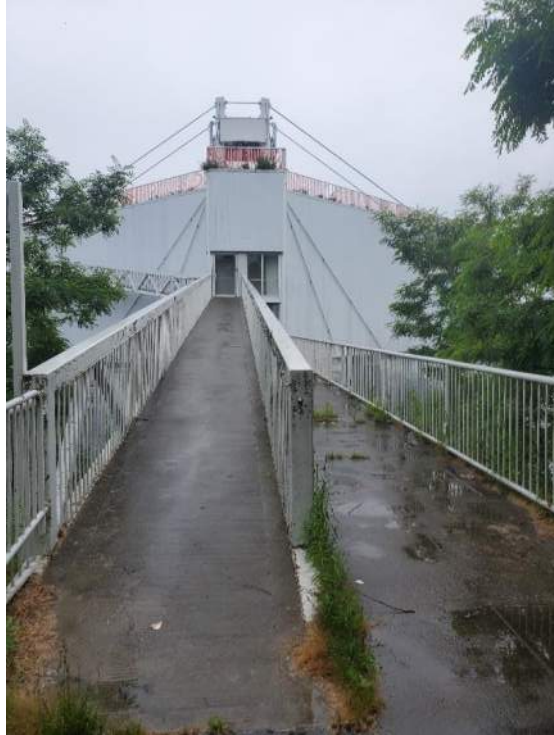
Figure 83: View, facing west towards Pod 5 (B92549-5), of the upper portion of Bridge 9 (B92573). July 5, 2022.
