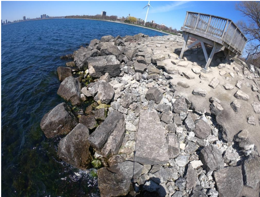
Figure 9: Damaged armour protection at west headland (Baird 2022-04-29)
