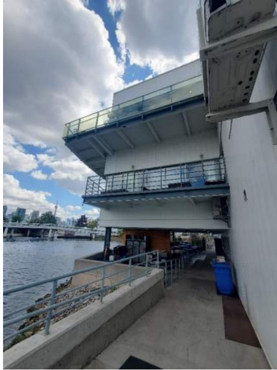
Figure 119: View, facing east, of Live Nation decks and lounges on the north side of the Budweiser Stage. July 12, 2022.
