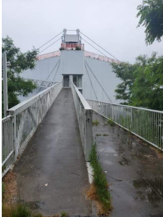
Figure 83: View, facing west towards Pod 5 (B92549-5), of the upper portion of Bridge 9 (B92573). July 5, 2022.
