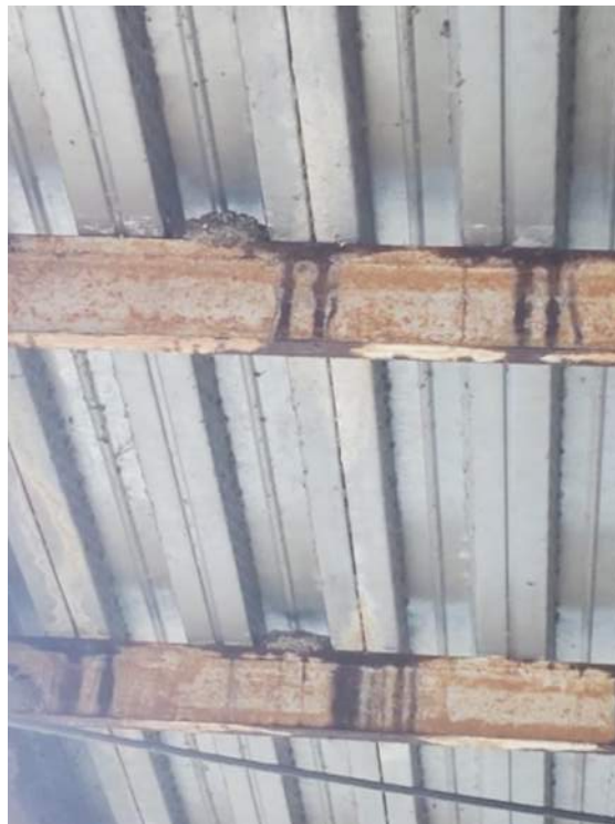
Figure 108: View of Barn Swallow nests on girders under Live Nation deck over water southwest of Bridge 2 (B2). June 23, 2022.
