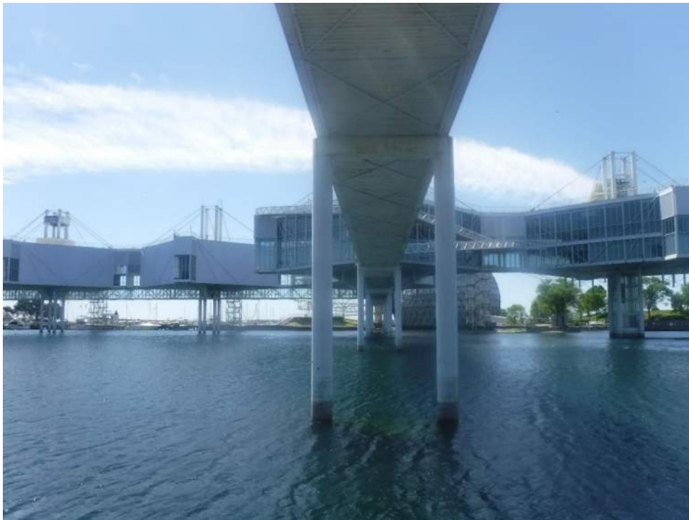
Figure 78: View, facing south of Bridge 10 (B92572) and the Pavilion Pods (B92549 - 1-5), which provide nesting areas for thousands of Cliff Swallows. June 16, 2021.
