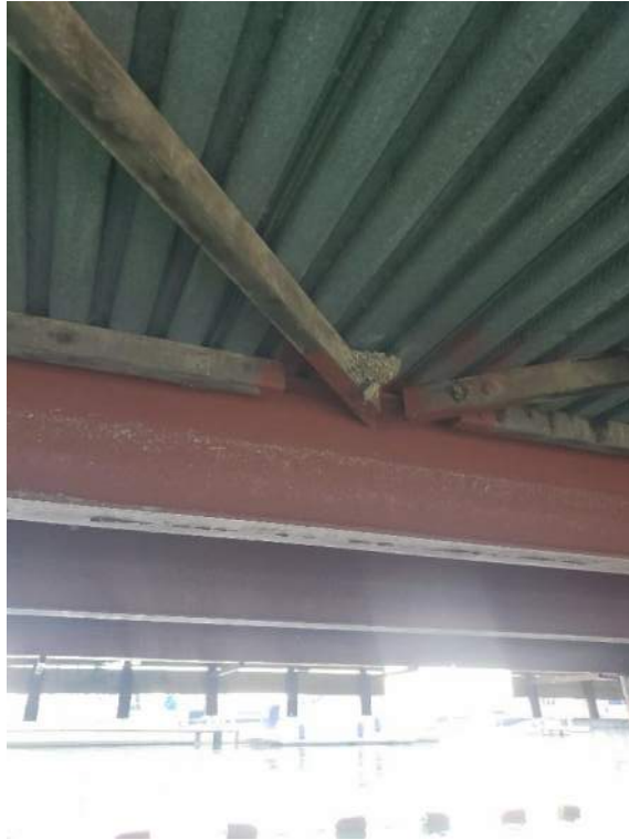
Figure 75: View of a Barn Swallow nest on the underside of Bridge 5 (B92575). October 11, 2022.
