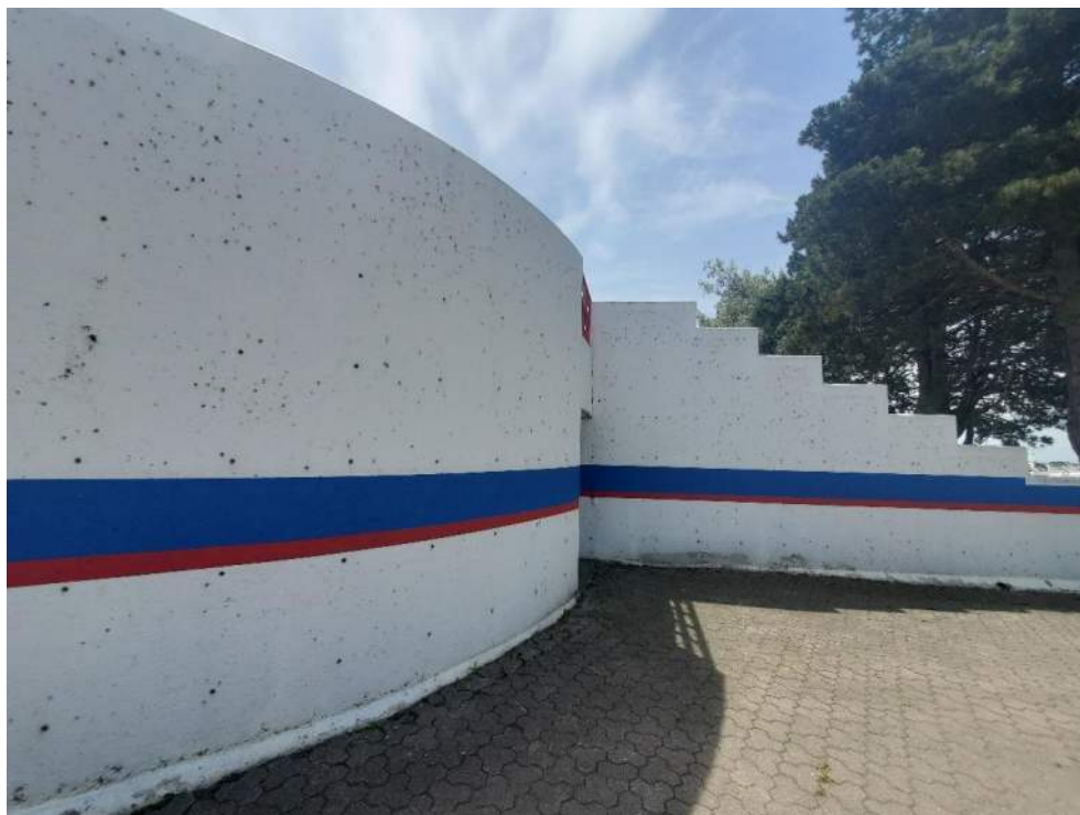
Figure 96: View, facing southwest, of exterior of the Marina East Washroom (B92554), and part of Bat Acoustic Monitoring Area #10.
