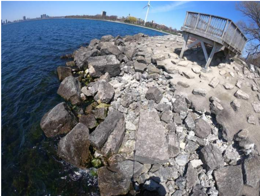
Figure 9: Damaged armour protection at west headland (Baird 2022-04-29)
