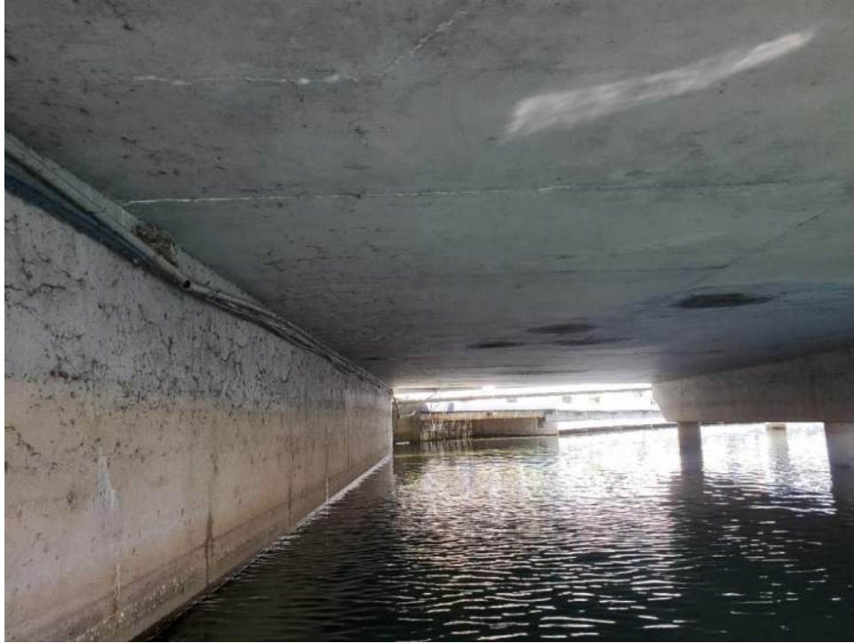
Figure 111: View, facing northwest, of the unnamed concrete bridge northwest of Bridge 2 (B2). June 23, 2022.
