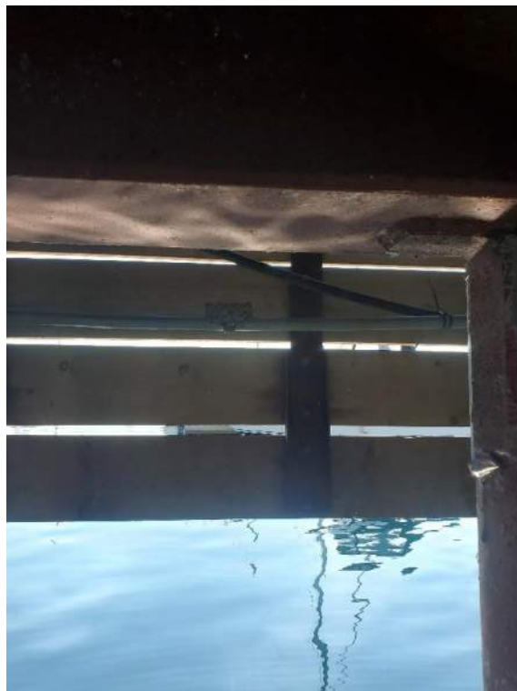
Figure 76: View of a Barn Swallow nest on a pipe underneath of Bridge 5 (B92575). October 11, 2022.
