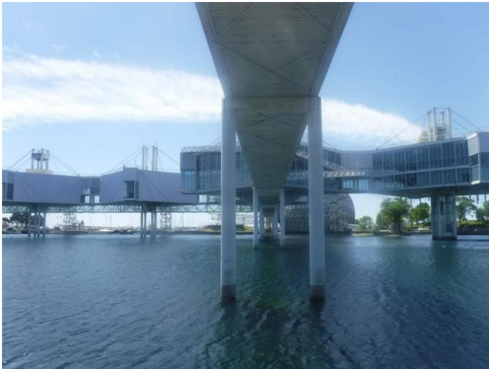
Figure 78: View, facing south of Bridge 10 (B92572) and the Pavilion Pods (B92549 - 1-5), which provide nesting areas for thousands of Cliff Swallows. June 16, 2021.
