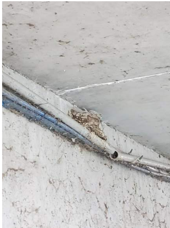
Figure 112: View of a Barn Swallow nest on cables in the unnamed concrete bridge northwest of Bridge 2 (B2). June 23, 2022.
