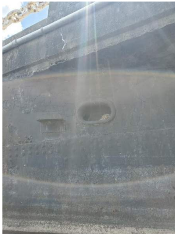
Figure 72: View of Barn Swallow nest in crevice within nook on the north side of the Breakwater (BW). June 23, 2022.
