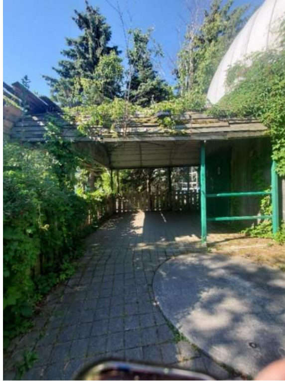
Figure 43: View, facing south, of covered entrance to the Interconnected Silos Complex at B92538-9. July 12, 2022.
