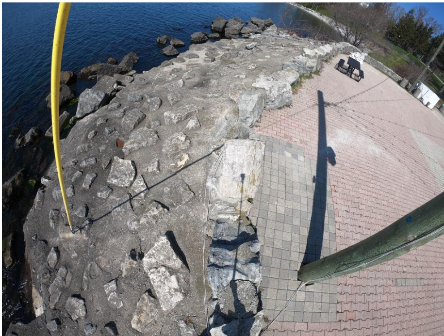
Figure 11: View of deteriorated grouted revetment at east headland (Baird 2022-04-29)
