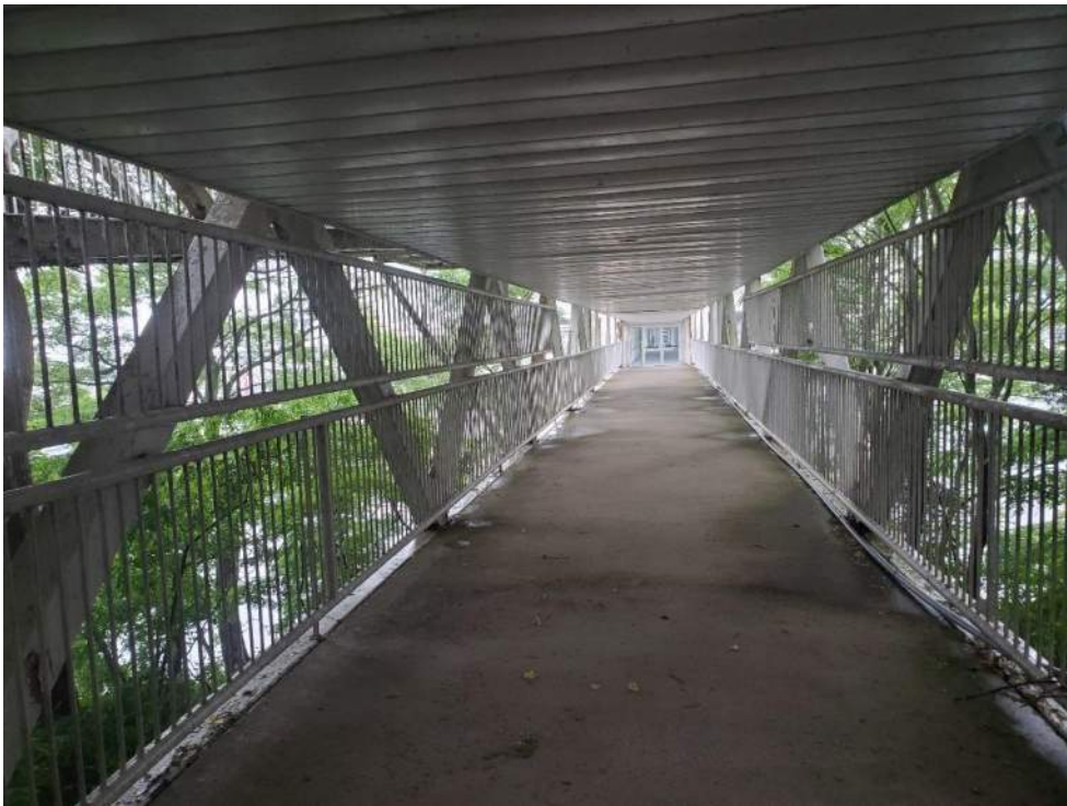
Figure 82: View, facing west towards Pod 5 (B92549-5), of the lower ramp of Bridge 9 (B92573). July 5, 2022.
