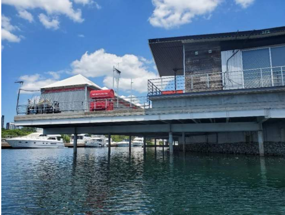
Figure 121: View, facing east, of the northwest decks over water on Live Nation grounds. The underside of the deck provides bird nesting habitat for Barn Swallows, American Robin and Common Grackle. June 23, 2022.
