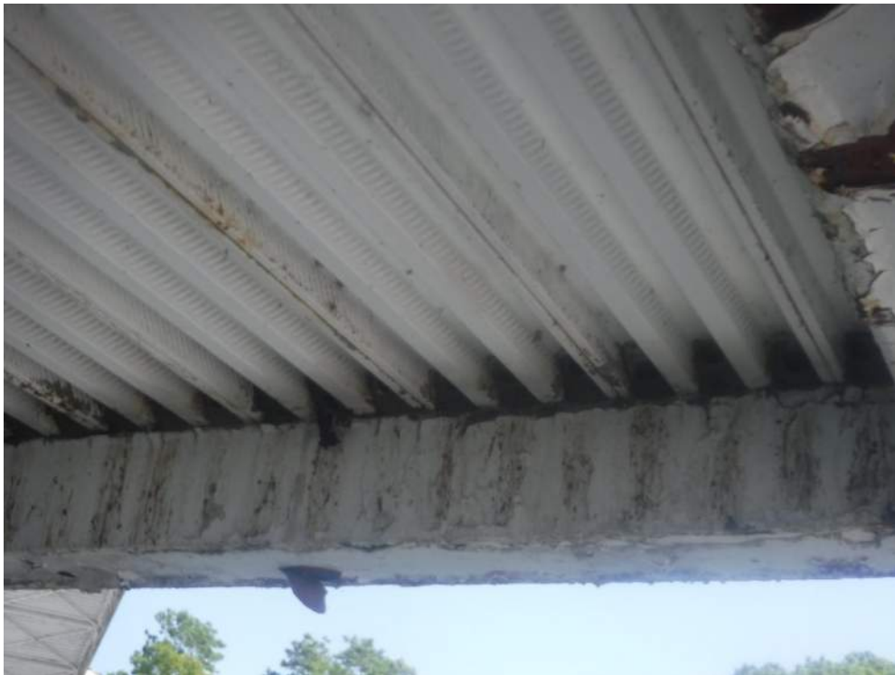
Figure 80: Close-up example of the metal grooves in underside of the Pavilion Pods (B92549 - 1-5) that provide Cliff Swallow nesting habitat. Cliff Swallow nests are visible in the end of each groove. June 16, 2022.
