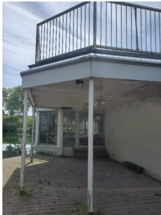
Figure 90: View, facing east, of a portion of the Marina North East Building (B92555) providing Barn Swallow habitat under deck visible in photo. June 20, 2022.
