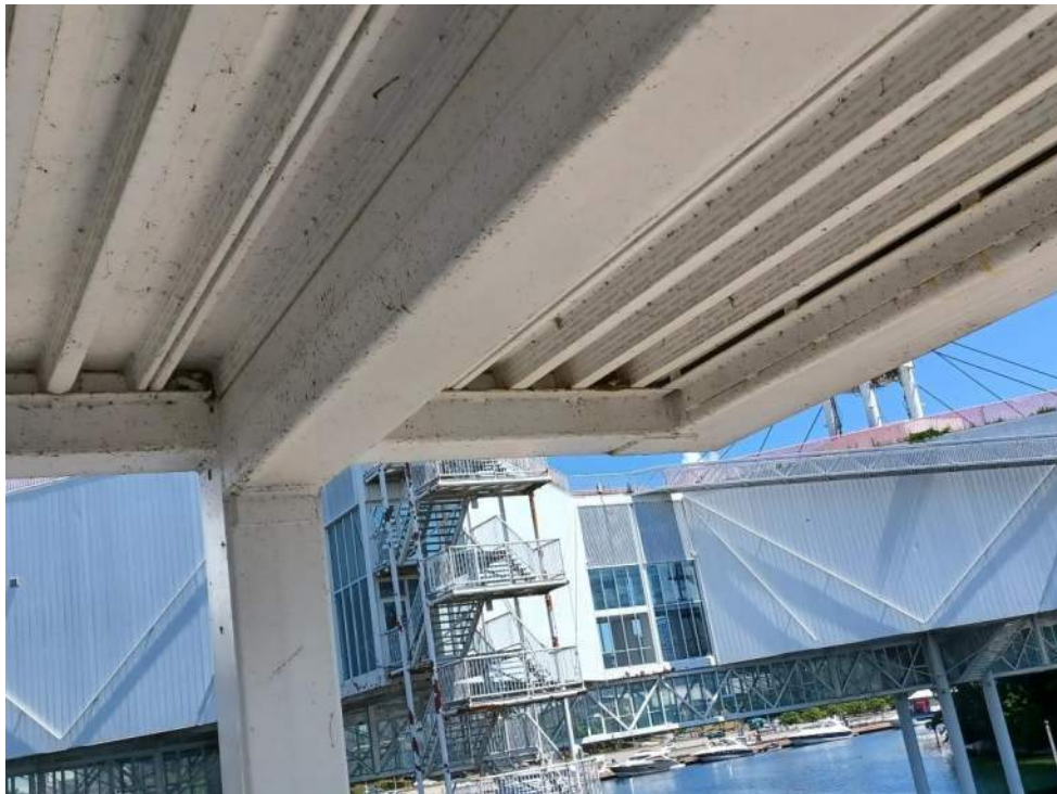
Figure 54: View of Cliff Swallow nests in grooves in underside of Secondary Tower Ramp Element 7 (SB7). June 23, 2022.
