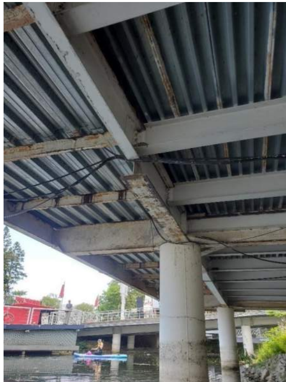
Figure 104: View, facing southwest, of the underside of the Live Nation deck over water providing Barn Swallow nesting habitat, with Bridge 2A (B2A) visible in the background. June 23, 2022.
