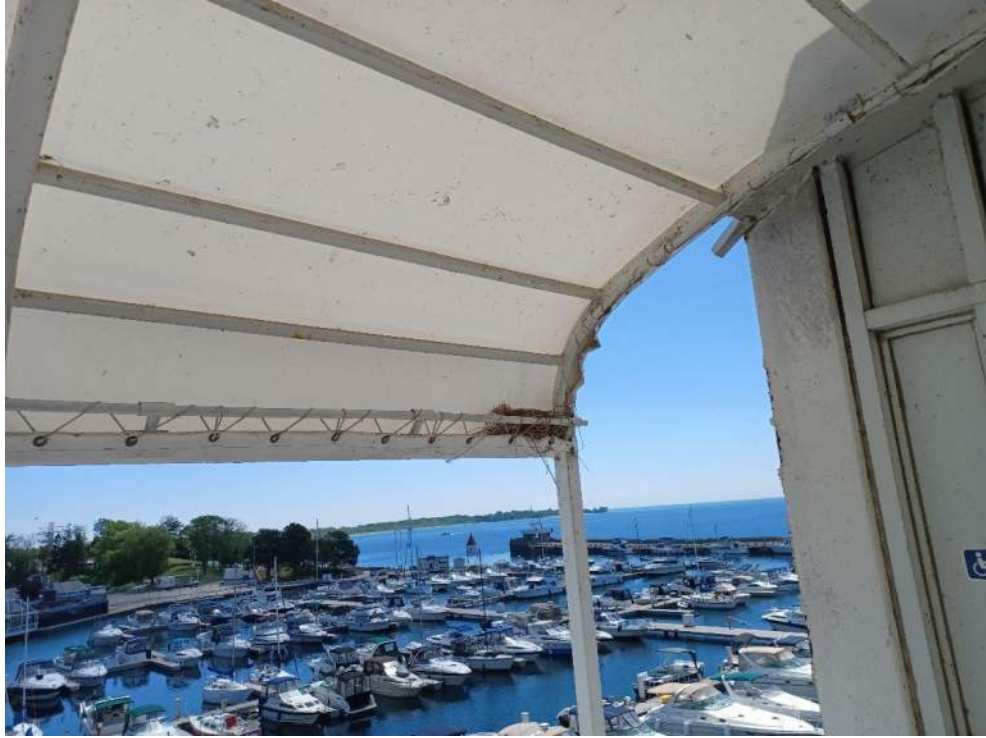
Figure 55: View of a partial, old, inactive American Robin nest on Secondary Tower Ramp Element 7 (SB7) awning. June 23, 2022.
