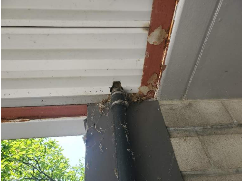
Figure 139: View of House Sparrow nest in the roof at the entrance to the Administration Building (B92578). June 20, 2022.
