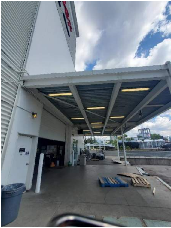
Figure 118: View, facing north, of the loading docks on Live Nation grounds. July 12, 2022.
