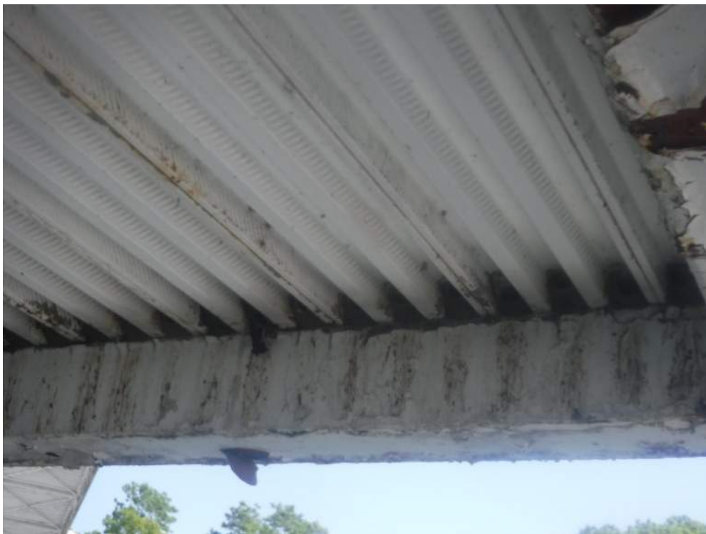
Figure 80: Close-up example of the metal grooves in underside of the Pavilion Pods (B92549 - 1-5) that provide Cliff Swallow nesting habitat. Cliff Swallow nests are visible in the end of each groove. June 16, 2022.
