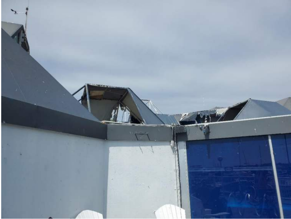
Figure 67: View, facing west, of the West Marina Village Building (B92550) roof providing Barn Swallow nesting habitat. June 20, 2022.
