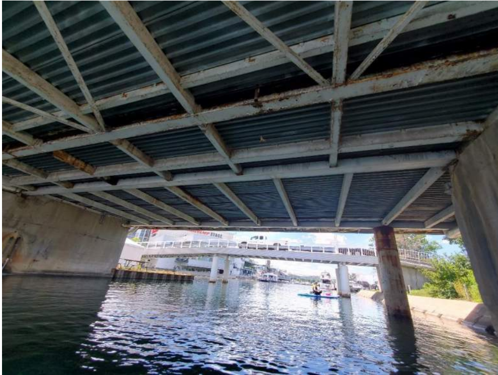
Figure 127: View, facing west, of the underside of Bridge 1 (B1) which provides Barn Swallow nesting habitat. June 23, 2022.
