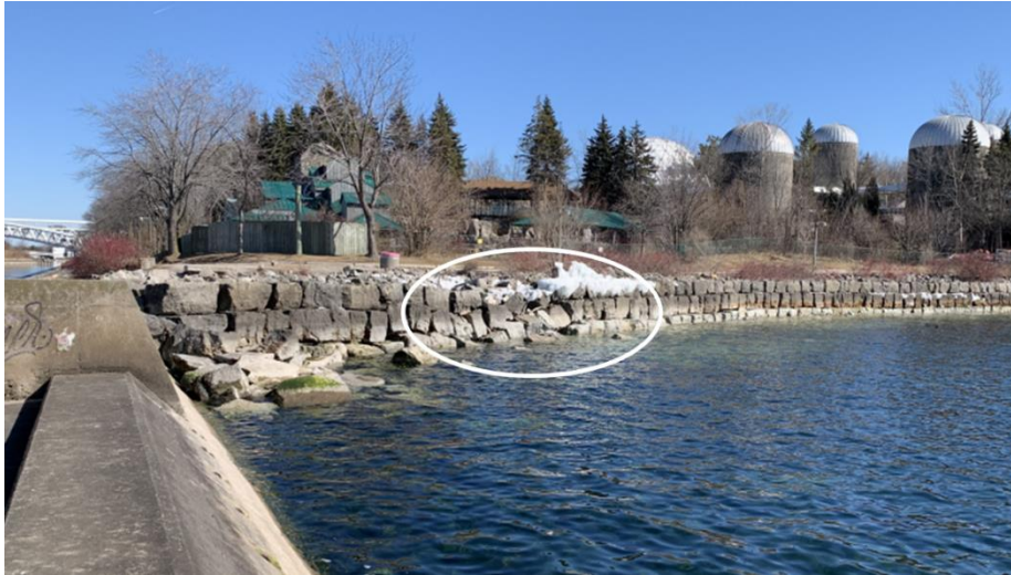
Figure 8: Collapsed portion of stacked armour stone seawall at west shore
