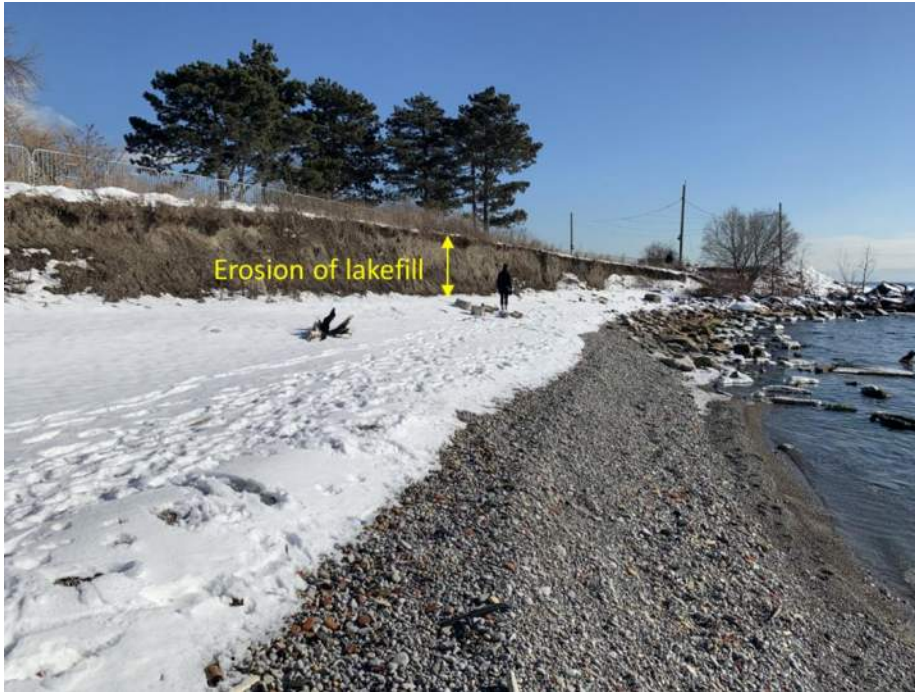
Figure 10: Significant erosion of lakefill at south shore (Baird 2021-01-30)
