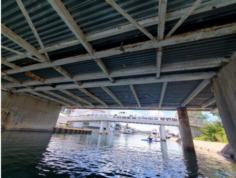
Figure 127: View, facing west, of the underside of Bridge 1 (B1) which provides Barn Swallow nesting habitat. June 23, 2022.
