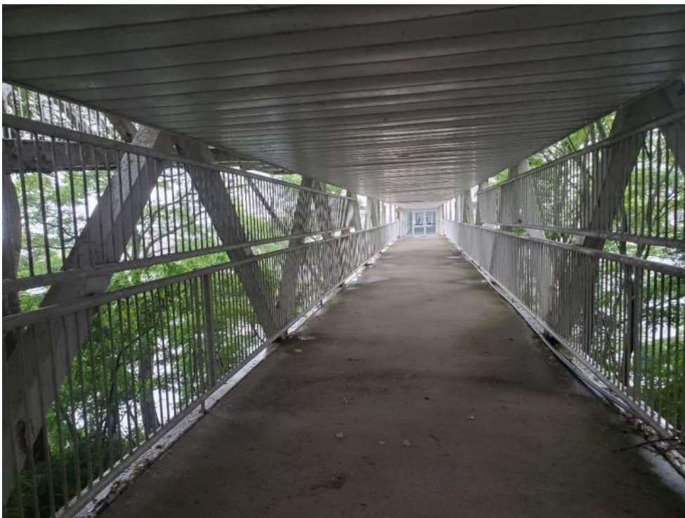
Figure 82: View, facing west towards Pod 5 (B92549-5), of the lower ramp of Bridge 9 (B92573). July 5, 2022.
