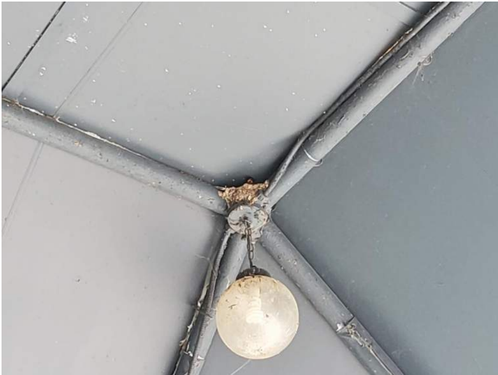
Figure 14: View of Barn Swallow nest on Commons Food Building (B92547). Barn Swallow visible sitting in nest. June 20, 2022.
