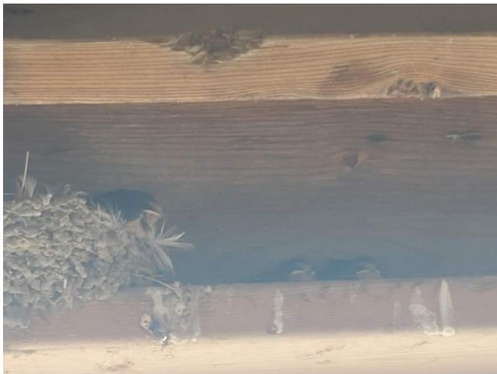
Figure 136: View of Barn Swallows and their nest under ledge of the roof of the Round Hut (B92563). June 20, 2022.
