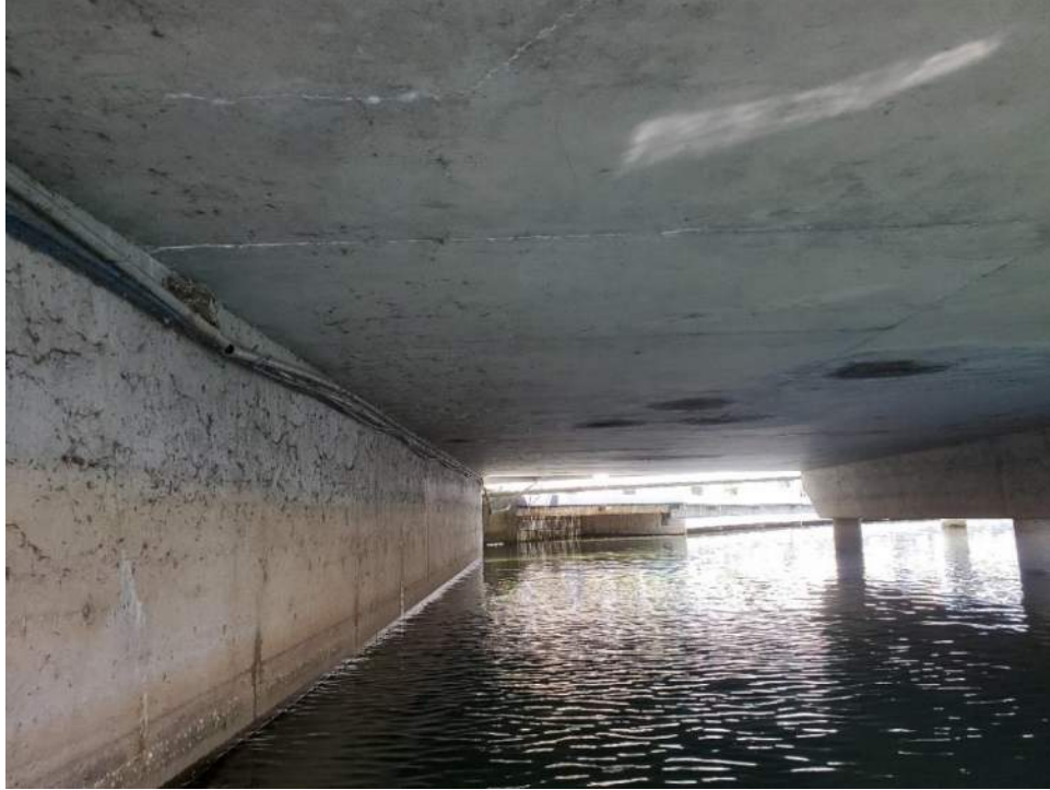
Figure 111: View, facing northwest, of the unnamed concrete bridge northwest of Bridge 2 (B2). June 23, 2022.
