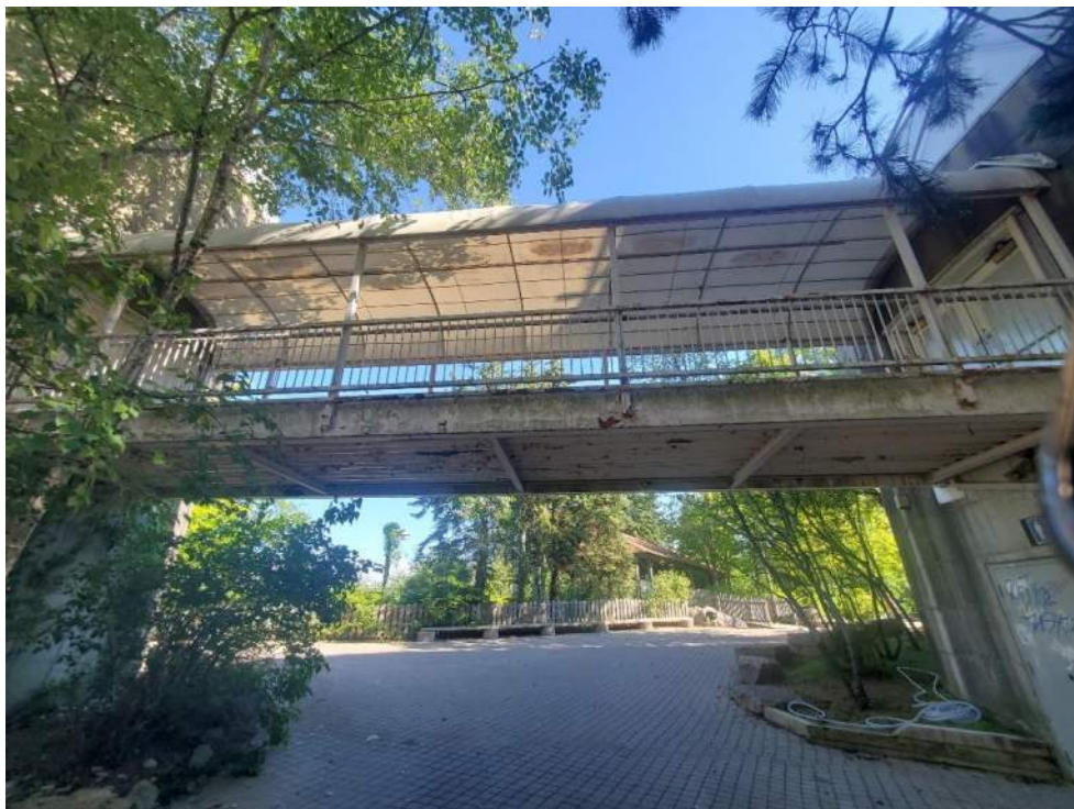
Figure 40: View, facing north, of the bridge between silos B92538-7 and B92538-8 in the Interconnected Silos Complex and of Landbird/Breeding Bird Survey Transect #5. July 12, 2022.
