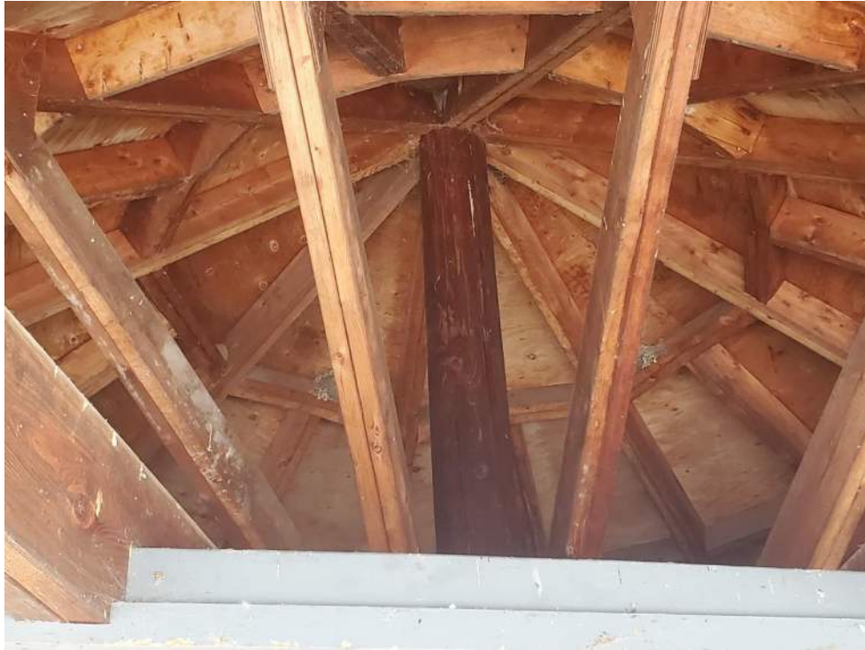
Figure 135: View of under roof of the Round Hut (B92563) showing. Barn Swallow nests in the rafters at the roof peak. June 20, 2022.
