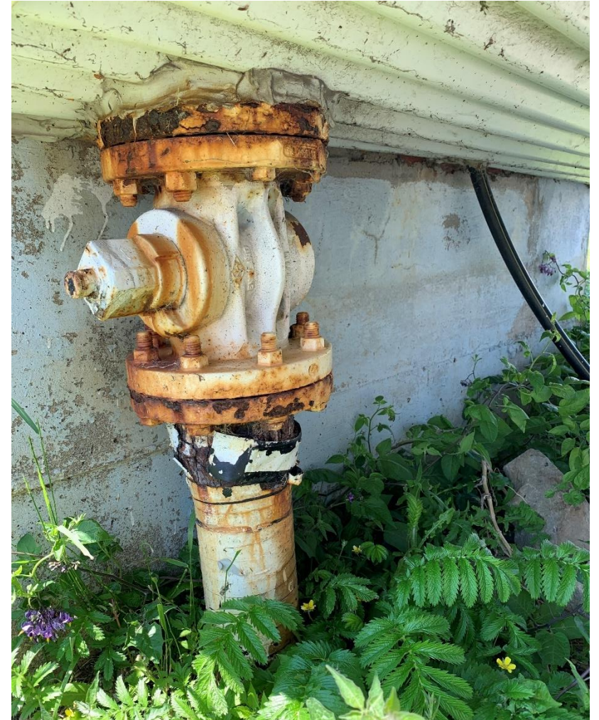
Corroded plug valve under Cinesphere bridge connecting to west marina.
